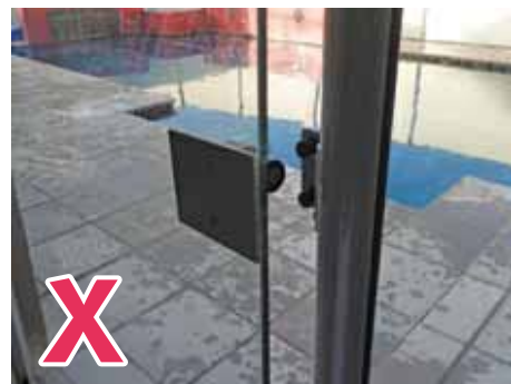
The gate or components may need to be adjusted or replaced to ensure the self-closing mechanism works properly.
