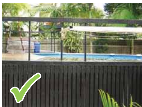
This deck bracing has been covered up with vertical palings less than 10 millimetres apart.
