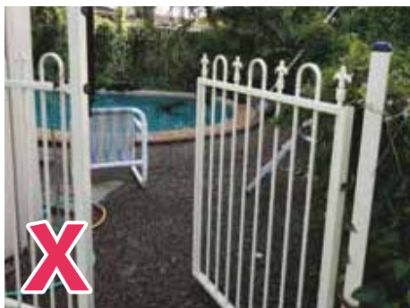
Inward opening gates must be modified to open outwards.
