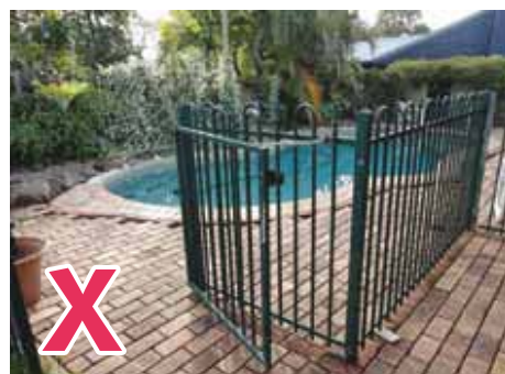
A gate cannot be tied or propped open when not in use and must self-close from any position.
