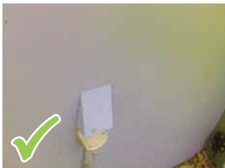
A power outlet has been shielded appropriately.
