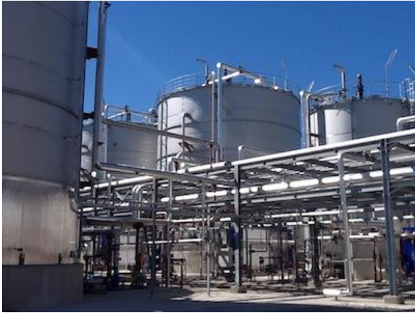
Figure 1: Beta Renewables Ethanol Plant in Crescentino, Italy
