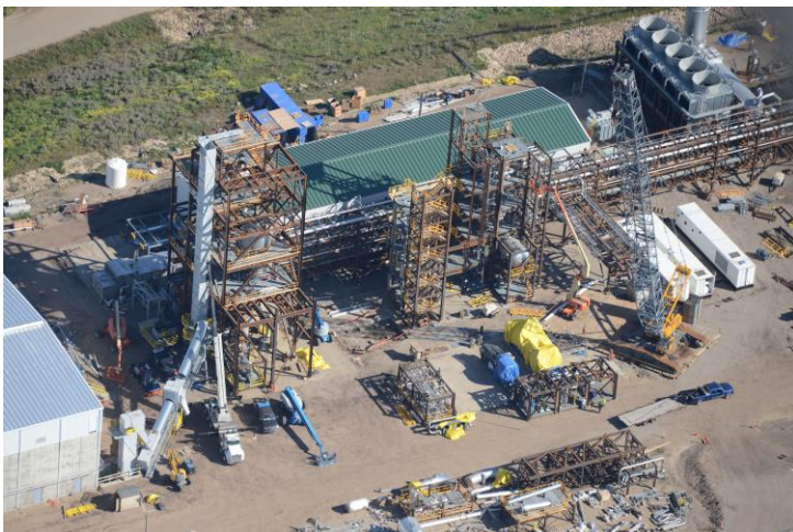
Figure 3: Enerkem MSW to Ethanol Plant in Alberta Canada
